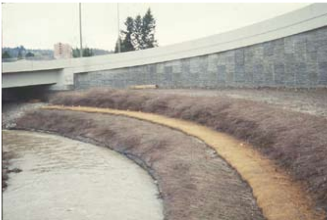
Figure TS14I-32 Completed VRSS ( Photo courtesy of Robbin B. Sotir & Associates, Inc. )
